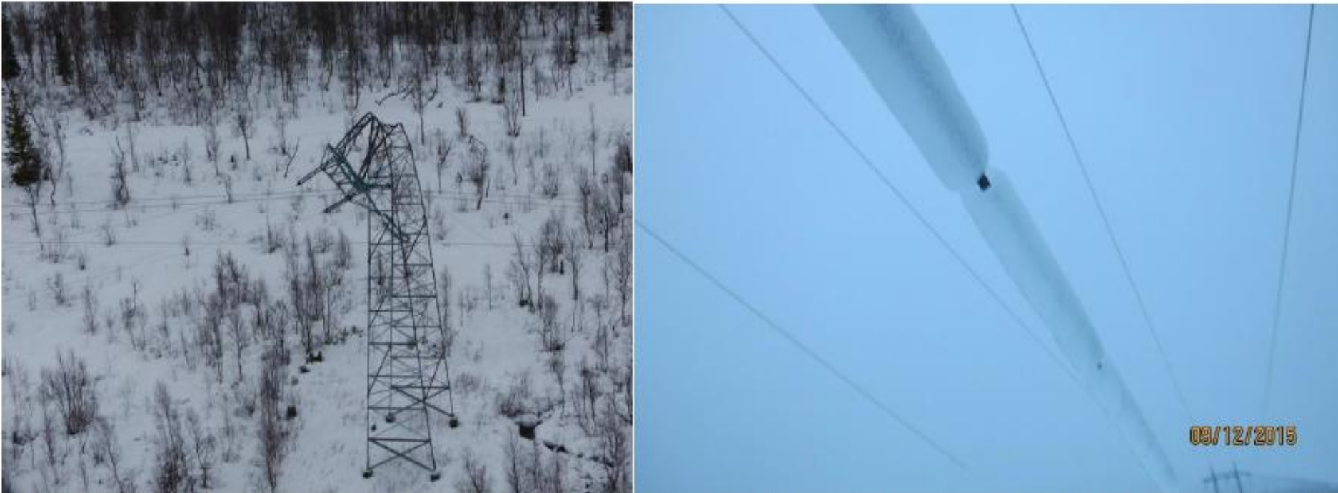
Figure 5-2 Left: Collapsed tower number 96. Right: Remaining ice on the broken earth wire, three days after the incident.
